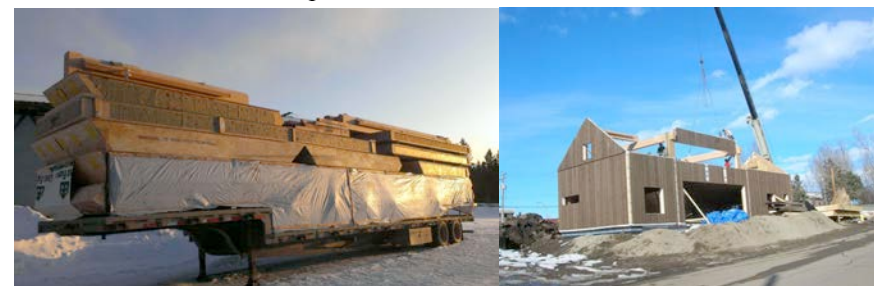
Figure 1 (a) Prefabricated thermal panels arriving on site. (b) Erection of the panels was complete within 10 days.
