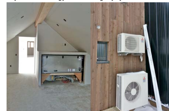
Figure 2 (a) Heat recovery ventilator installed in upper level closet. (b) Outdoor installation of air source heat pumps.
