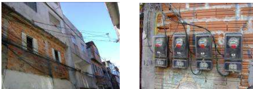
Figures 14 e 15 On the left, the precarious electricity grid running in front of windows in favela Morro da USP . On the right, the multiple electricity meters installed in one residential building.
